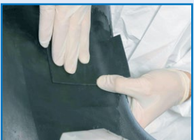
As there is no need for curing, you are now ready to tackle the front of the repair
