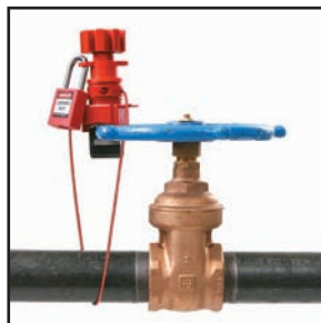
Use cable attachment to lock out gate valves
