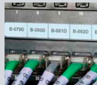
Patch panel and terminal block ID
