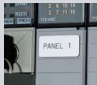
Control panel labels
