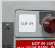
Asset and equipment ID
